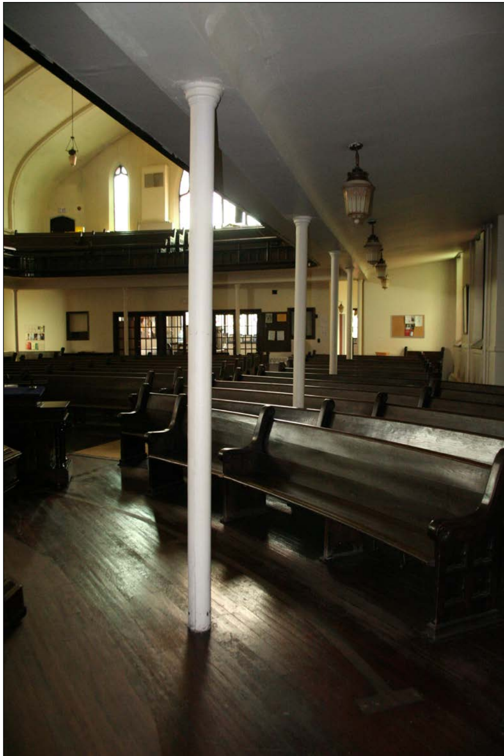
Plate 22 – Augustine United Church, 444 River Avenue, east side gallery support columns, 2007. ( M. Peterson, 2007. )
